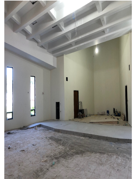
The renovated Chapel will seem airier, with the sanctuary extended forward, new stained glass windows on the side, and the balcony removed.
