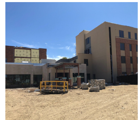
The front entrance is getting a facelift. To the right is the renovated building of four stories of apartments, along with offices on the 1st floor.
